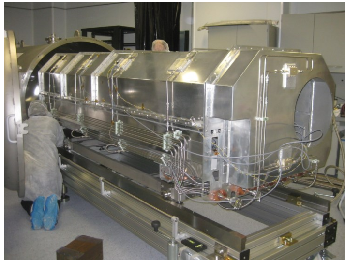
Figure 4. View of the in-vacuum cooling hardware, mainly the RadSh, outside the VV.
